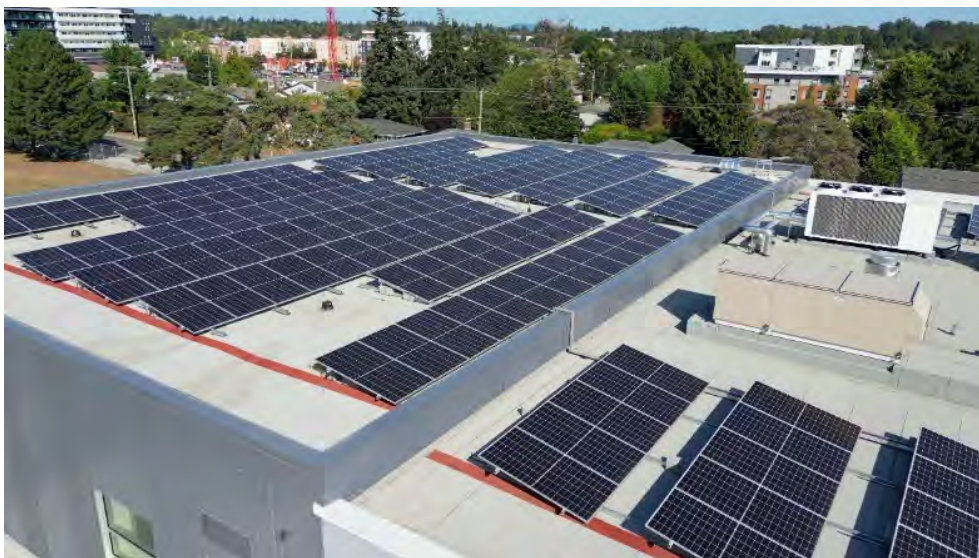
100kW photovoltaic array on the roof of Cedar Hill Middle School (upgradeable to 350kW.).
