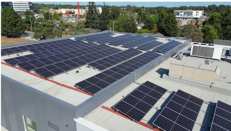
100kw photovoltaic array on the roof of Cedar Hill Middle School (upgradeable to 350kW.).
